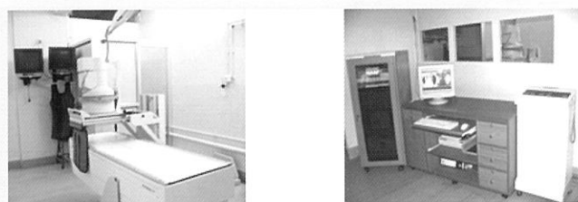
Fig. 18 DMIS installed at BARC Hospital (left- imaging unit and right – controls)
