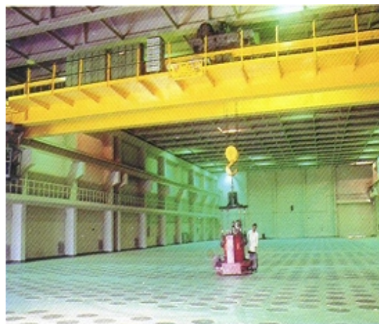
Fig. 7 View of air cooled Solid Storage & Surveillance Facility, Tarapur
