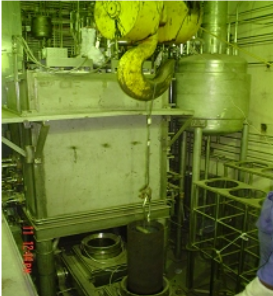
Fig. 6 Compact ceramic melter installed at AVS, Tarapur
